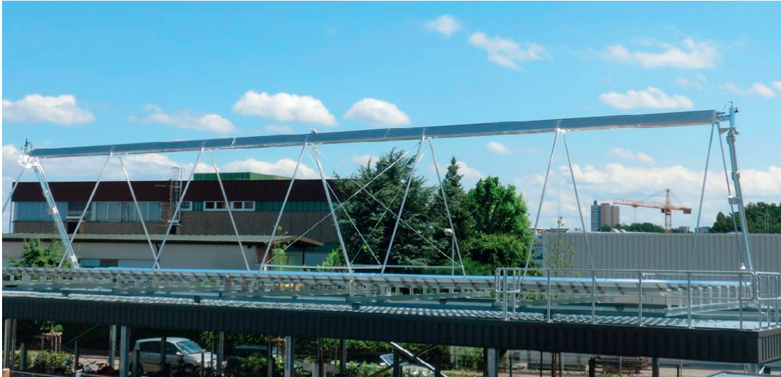
Fig. 4. Collector string of pilot installation
