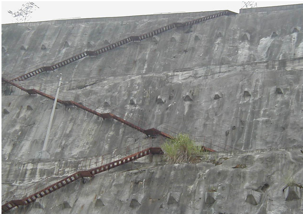
Fig. 8. Photo of anchor cables laid out at the high slope of double-lane five-step ship lock.
