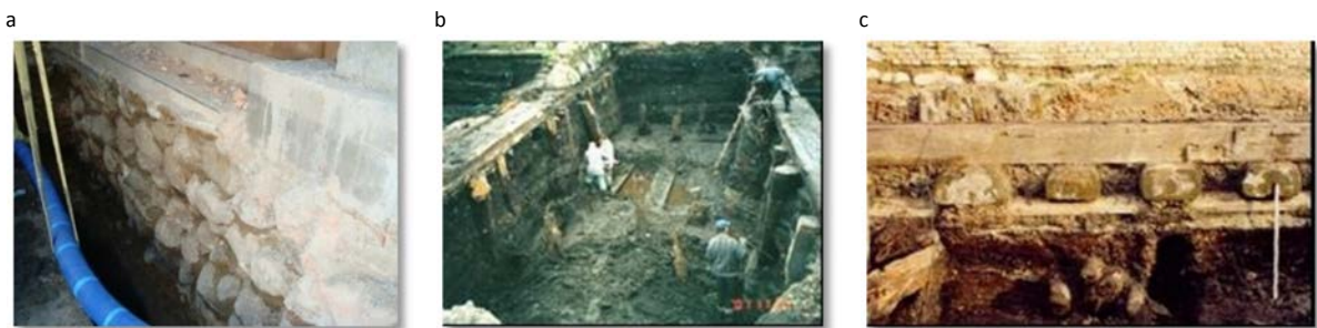
Fig. 1. View of foundations: (a) historical building in Olsztyn at Staromiejska Street; (b) old granaries at Basztowa Street in Gdańsk; (c) old granaries at Chmielna Street in Gdańsk.
