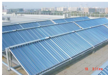
Fig. 1. Photo of solar collector array
