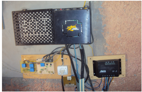
Fig. 3: Photo of the Whisper charge controller and hybrid system controller
