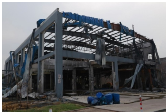
Fig. 1. The burned-out workshop.
