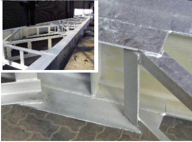
Fig. 5. Cracks on a truss after hot dip galvanizing
