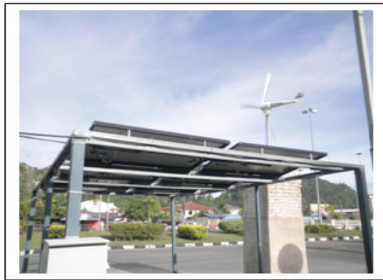
(b) PV array and wind power generation
