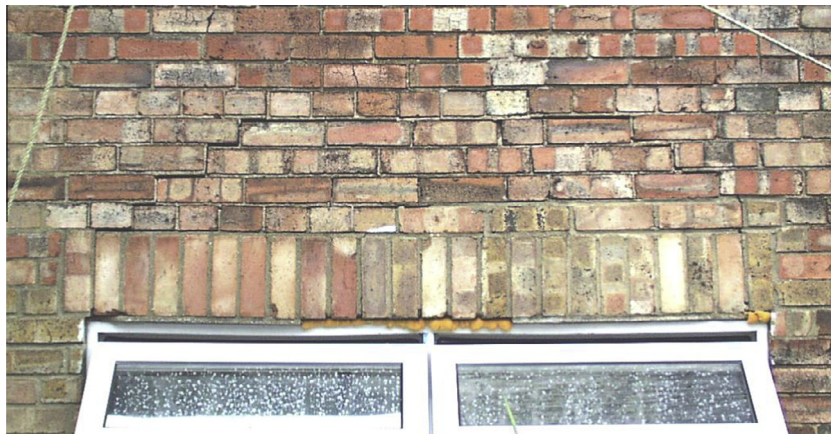
Fig. 2. Damage in a masonry wall above a window opening (Courtesy of Bersche Rolt Ltd).
