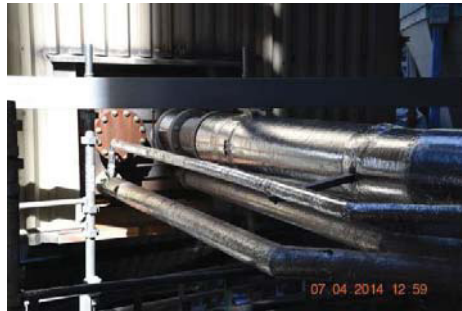
Fig. 1. Flue gas supply
