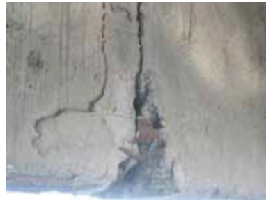
Fig.3. Crack at the wet joint.
