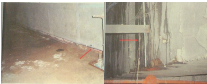
Fig. 2. Leakages due to poor workmanship at AHU room above Operation Theatre (a) The improper wall plastering at AHU room, the water can enter through the wall (b) The leakages sign at the beam under the AHU room slab
