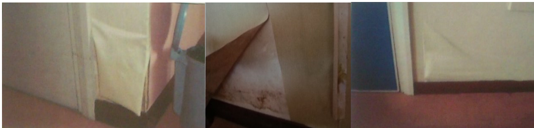
Fig. 7. Peeling of wallpaper at level 7 and 6 Ward Block due to waterproofing failure
