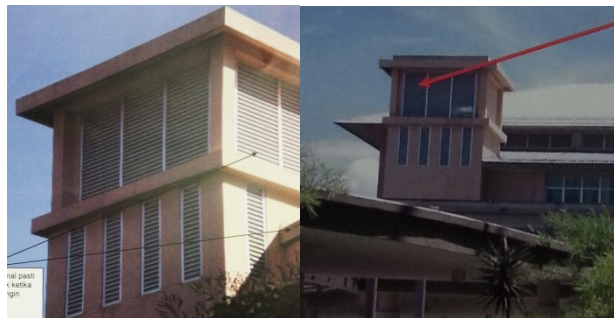
Fig. 1. Cause of leakage: rainwater enters through the louvres due to shortness of awning
