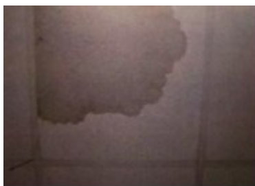
Fig. 3. Watermarks on ceiling due to water drop (condensation) from Exhaust Fan Ducting system at Pharmacy Store
