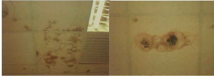
Fig. 4. Condensation cause dampness and mould growth at the Rehabilitation Unit's ceiling
