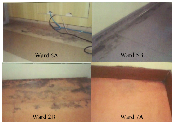
Fig. 5. Black staining and dampness on floor finishes at 7 Storey Ward Block due to water seepage from toilet area
