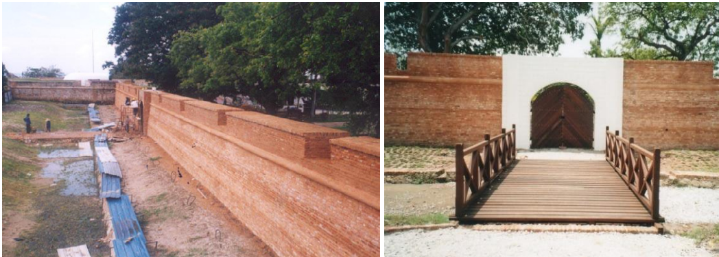
Figure 5: The reconstruction of west wall Fort Cornwallis (2001) was based on several references including the old survey map, photographs and archaeological findings. Reconstruction of the west wall involved thousands of salvaged red clay bricks supplied from abandoned old shop houses in Penang built between 1892 and 1928. The salvaged red clay bricks were laid down according the original brickworks.
