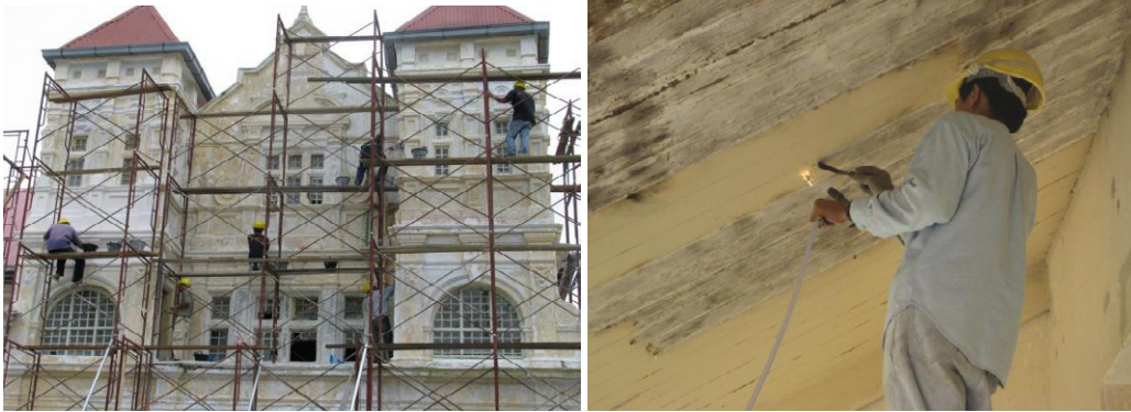
Figure 4: Paint's scrapping to reveal the original colour of exterior wall Taiping Museum (Left) and paints scrapping using burning technique.
