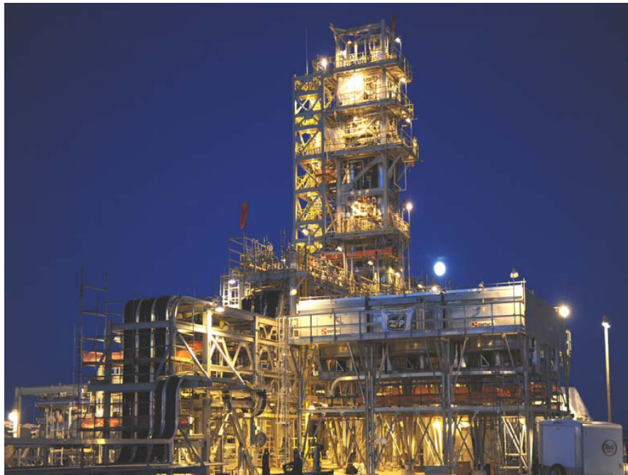
Figure 7. The CFZ™ Commercial Demonstration Plant.
