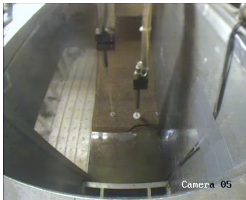
(a) Cracks at the water level of 146.9 m.
