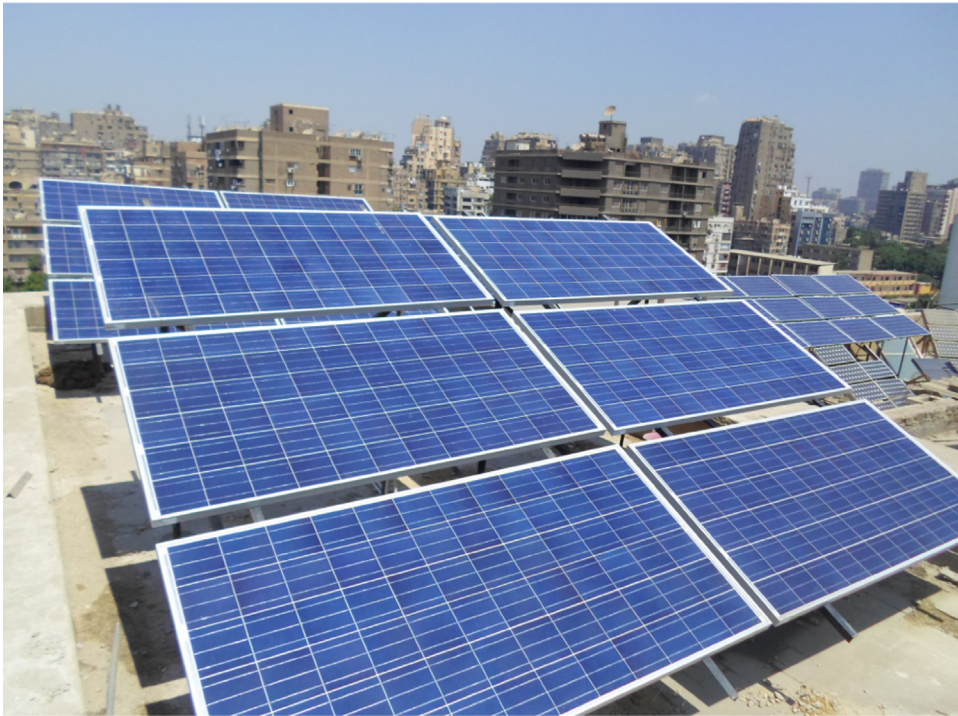
Fig. 1. Photo of the installed PV array at roof top of ERI site.
