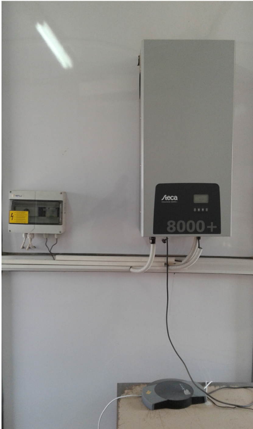
Fig. 2. Photo of the considered inverter.
