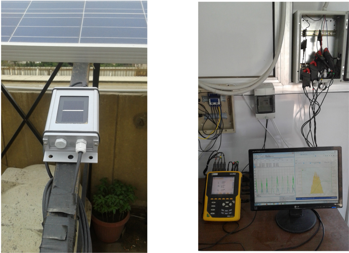
Fig. 3. Photo for the used monitoring and data acquisition system.
