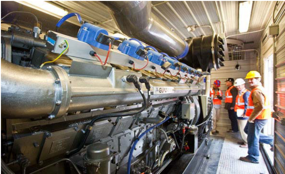
Fig. 1. Methane monitoring equipment
