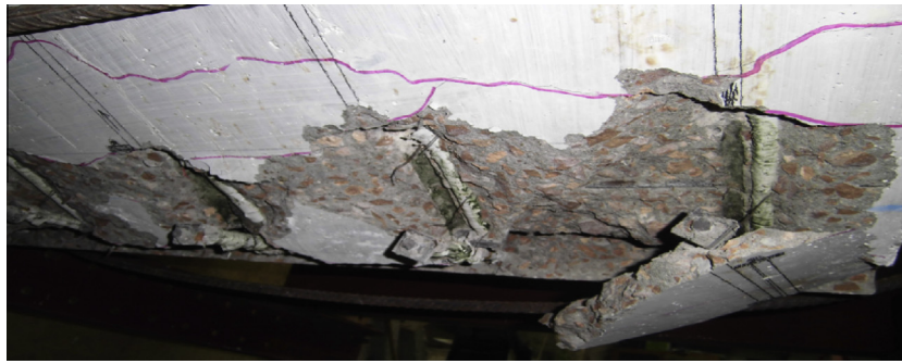
Figure 5 Brittle failure of the lap splice on the bottom of slab AS-4 (debonded bars).
