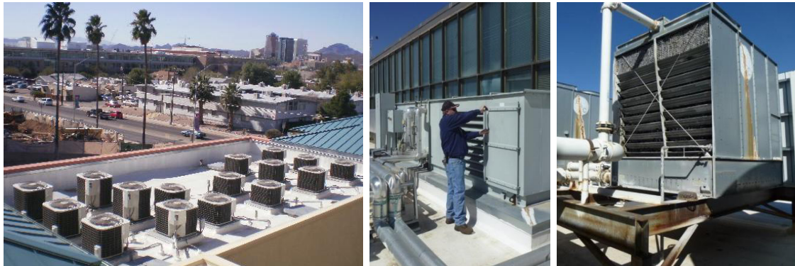
Fig. 4 (left) La Aldea split heat pump HVAC system, (Middle) CAPLA chilled water units, and roof-top cooling towers at the USB Building.
