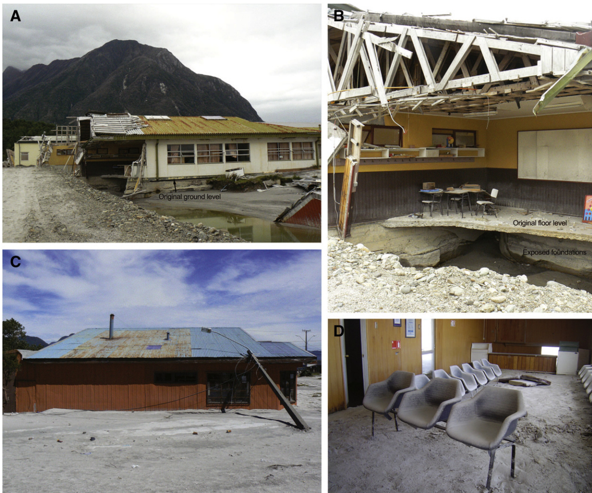
Fig. 12. (A, B) Extensive damage to a school in Chaitén town, Chile from a lahar after the 2008 eruption of Volcán Chaitén. Two exterior walls have been completely removed and the ground around the foundations has been scoured. (C) Burial of a building, up to window level, in Chaitén town from a lahar after the 2008 eruption of Volcán Chaitén. A power pole is also damaged. (D) A building in Chaitén town, inundated by a lahar after the 2008 eruption of Volcán Chaitén. Photos: G Leonard.
