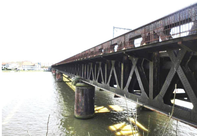
Fig. 1. Global view of the Eiffel bridge over the Adour river (photography taken in 2013).
