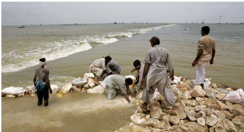
Fig. 8. Pakistani workers pile rocks along the embankment surrounded by heavy floodwater in Shadadkot, southern Pakistan – photo by AP published in Dawn , August 26, 2010.
