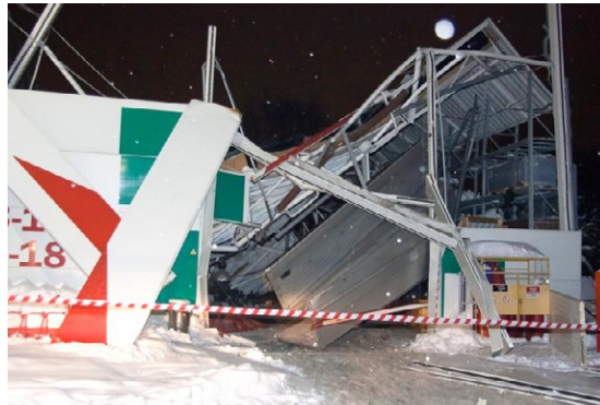
Fig. 4. A supermarket roof collapsed under snow load in 2012, by Girts Gertsons. Retrieved from the http://girtsons.blogspot.com
