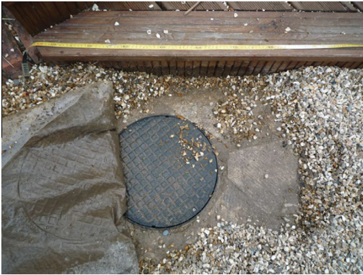
Fig. 11. Exposed drain cover.
