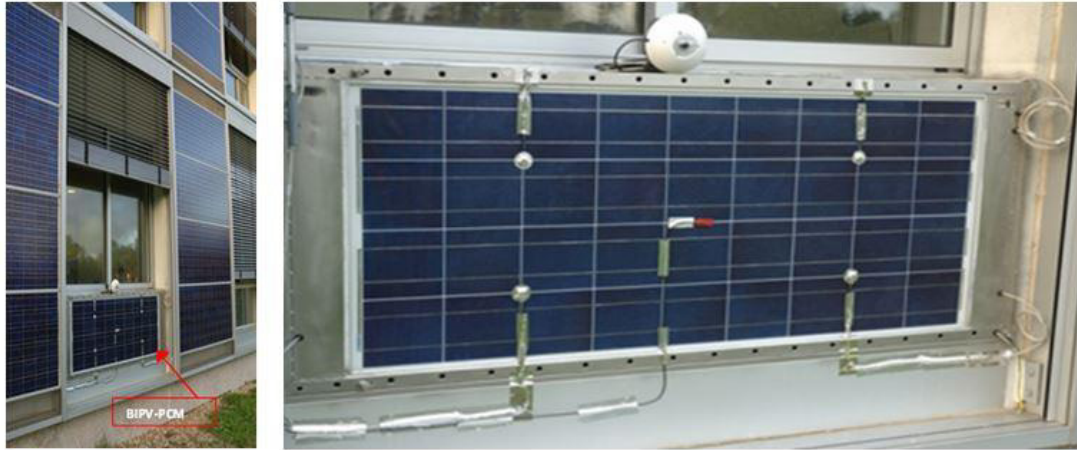
Fig. 3. Views of the prototype installed on the SolarXXI main façade.
