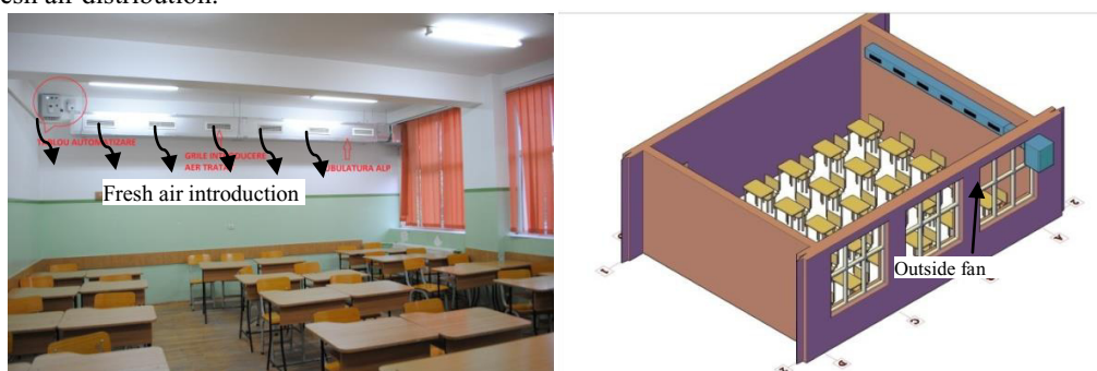
Fig. 2. Classroom S8 with the ventilation system mounted in the back of the classroom and 3D view
