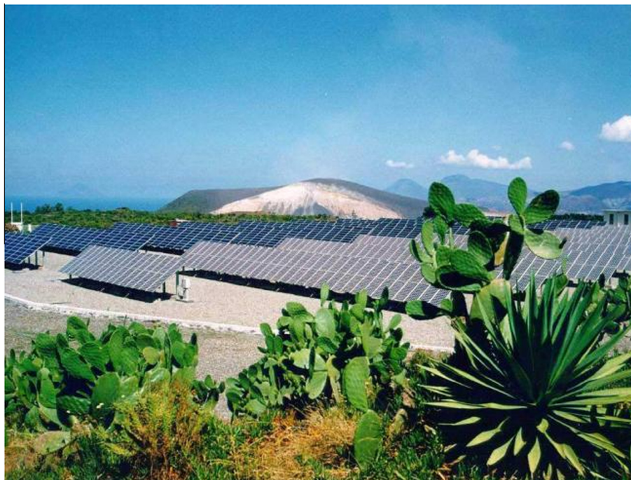
Figure 1. Two PV fields (80 kW the one on the right; 100 kW the other) comprised of different crystalline silicon solar modules installed in the island of Vulcano, Sicily.
