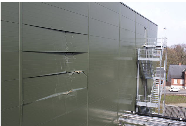
Fig. 4. The tank rose nearly vertically in the air, and the base of the tank rose higher than the 19-m tall green building. While descending, the tank impacted and deformed the building's exterior wall panels. (Photo courtesy of F.H. Hedlund.)
