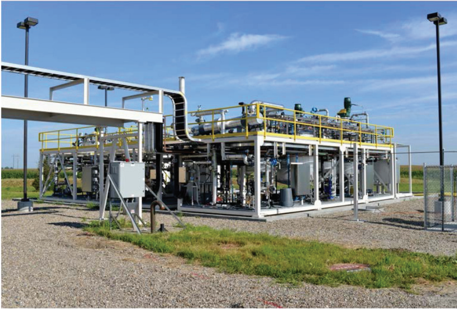
Fig. 3. Iowa State University's vegetable based bioadvantaged polymer pilot plant facility.
