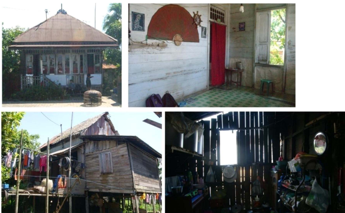
Fig. 2. Investigated houses condition. Exterior and Interior of Investigated House B (Left). Exterior and Interior of Investigated House F (Bottom). (source: Field Survey (2014)).
