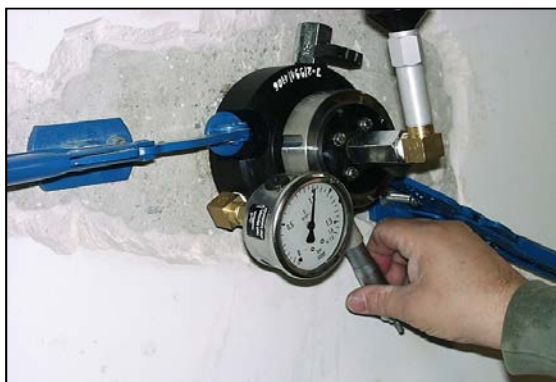
Fig. 2. View of GWT chamber during measurements
