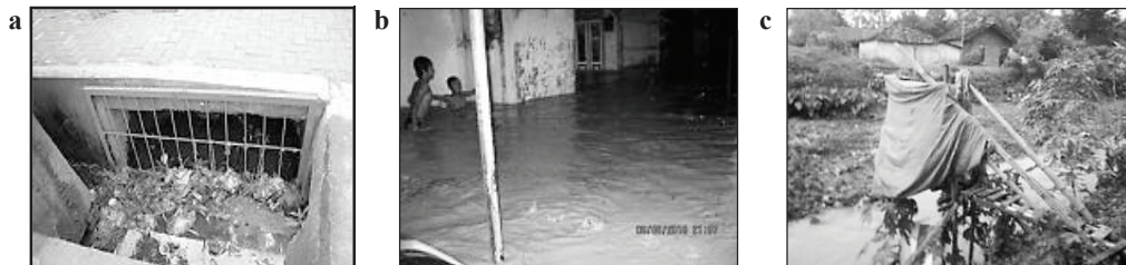
Fig. 5. (a) Garbage blocking drainage system; (b) Flood in housing areas; (c) Inadequate sanitation system.
