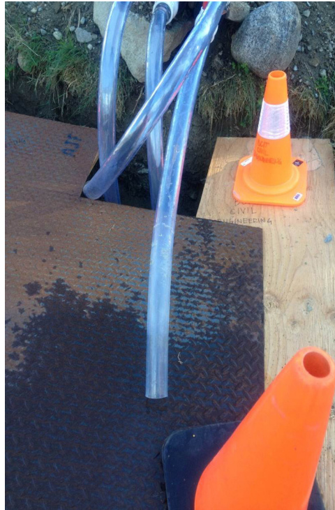
Photo 3. Downstream end of pipes feeding into a collection chamber.
