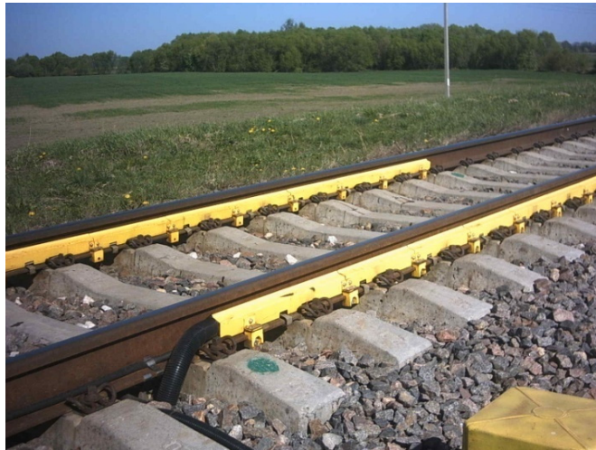
Fig. 1. Wheel impact load detector.
