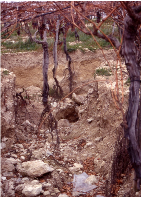
Fig. 4. The total lack of practices to mitigate water runoff, accelerate rill and gully erosion that reduces soil fertility and organic carbon stock.
