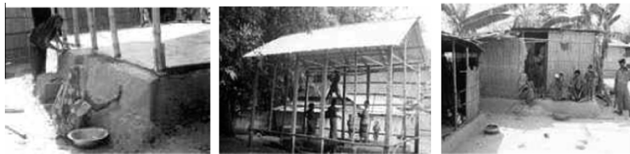
Fig. 3 The construction practices advocated by the NGO ‘practical action’ and targeting flood resilient houses in Bangladesh ( http://practicalaction.org/practical-action-bangladesh-1 : accessed on 17th of April 2013).
