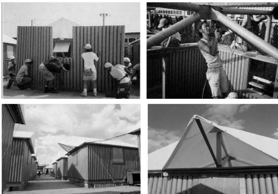
Fig. 8 (Above) The easy and fast assembly of the 'blog house' cardboard tubes. (Below) The roof tenting material and the operable hatch of the 'blog house' [11].
