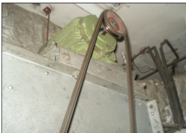
Fig. 2. 2.2 kW motor used for AC chiller plant.
