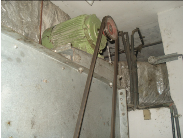
Fig. 3. 1.6 HP motor used for water treatment.
