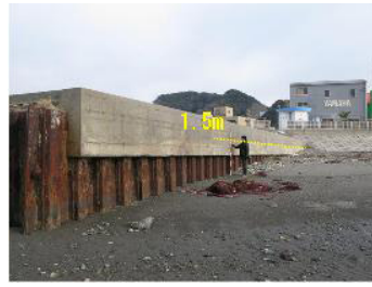
Fig. 14. Exposed foundation of left bank jetty .
