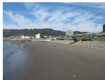
Fig. 8. Eroded beach of a gentle slope and scarp formation on gently sloping revetment.
