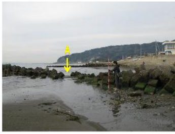
Fig. 13. Opening in left bank jetty caused by subsidence of concrete blocks.
