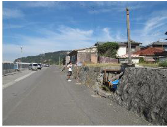
Fig. 9. Gaps in old seawall left on landward side of road.
