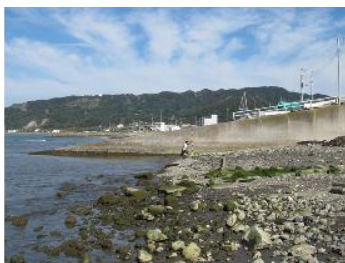
Fig. 7. Isolated concrete slope for boating and eroded beach.
