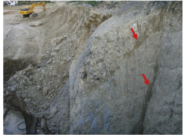
Fig. 10. Seepage through secondary joints along which the sliding occurred.
