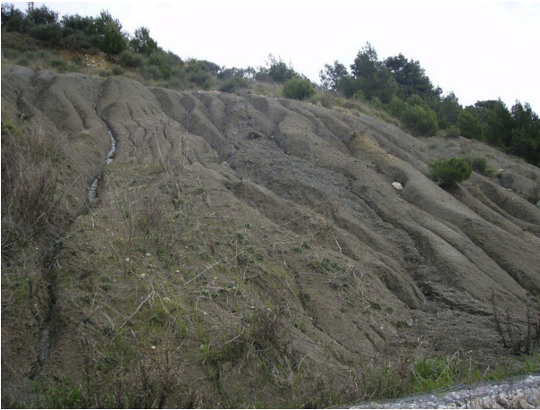
Fig. 1. Marl degradation on the surface of a cut slope on the Adriatic Highway (Podstrana municipality).
