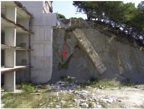
(c) Seepage through secondary joints (2006).
