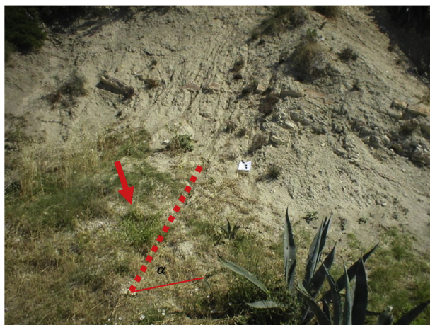
Fig. 6. Measured inclination of weathered marl deposited at the bottom of the slope (arrow), inclination range \alpha = 31^\circ\text{--}38^\circ .
