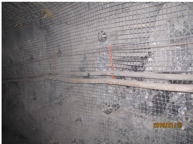
(a) Sidewall in the narrow coal pillar.
