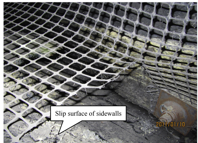
(b) Slip phenomenon of sidewall in the narrow coal pillar.
