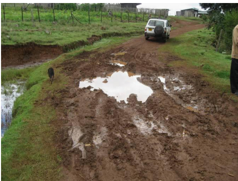
Photo 6. Road condition before maintenance at demonstration site in Kenya.
