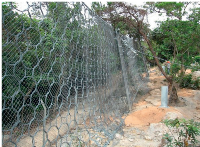
(a) Flexible barrier at the toe of a natural hillside.
