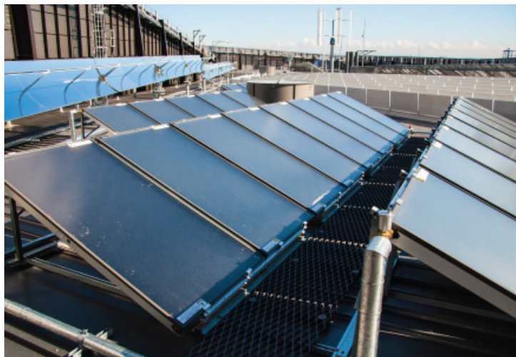
Figure 4. View of parabolic trough (rear) and flat plate collectors (front) on the roof of the UTS building. Source: J. Osborne
