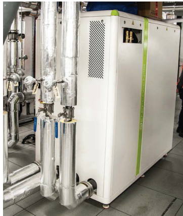
Figure 3. Eneftech ORC generator 010GRE-01. Source: J. Osborne
