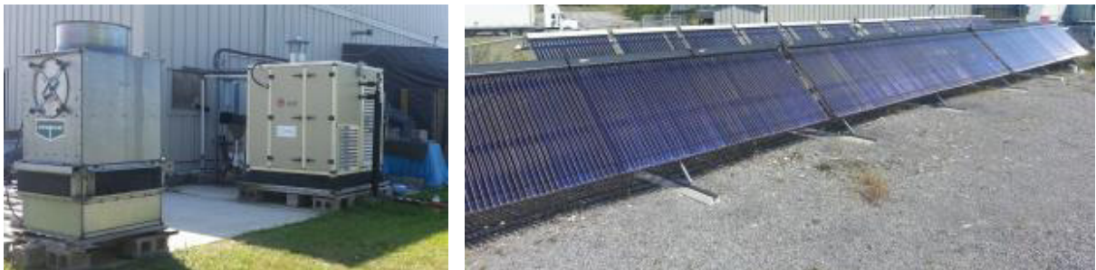
Fig. 1. (a) Liquid desiccant air handling unit and cooling tower as installed at Queen's University; (b) Photo of the solar thermal collector array
