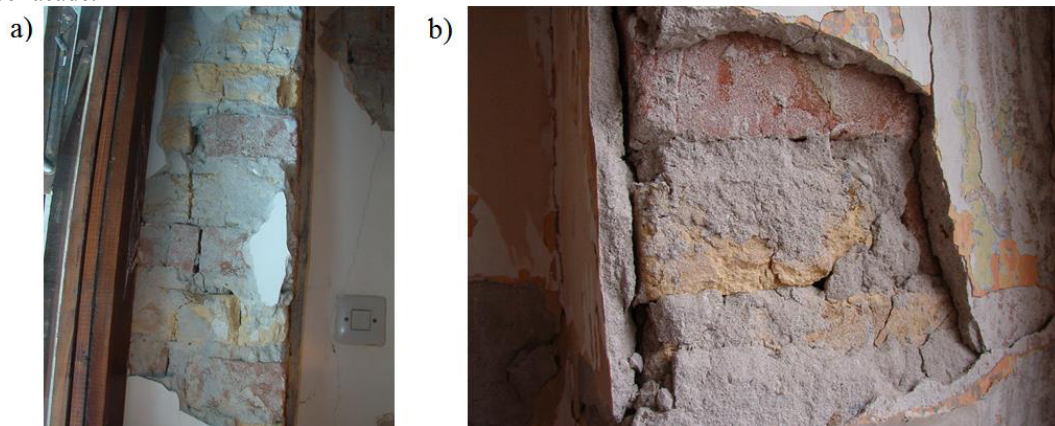
Fig. 4. a) Damages of basic material, b) Unequal thickness of the vertical and horizontal joints in wall
