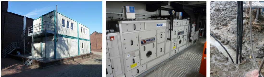
Fig. 1. Test facility, air handling unit and BHX.
