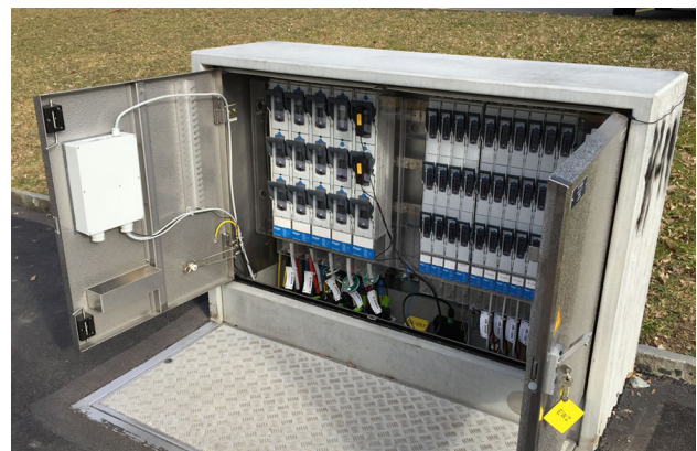
Fig. 8 GridBox installed at a distribution cabinet
