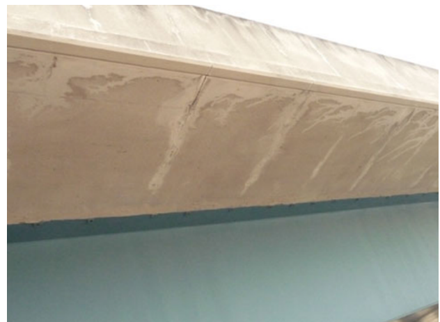
Fig. 1 Pictures of deck cracking in Fort Lauderdale, FL.
