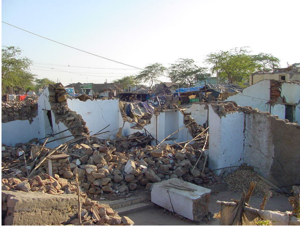
Fig. 44 Destroyed masonry houses in the village of Maliya (photo: C. V. R. Murty)
