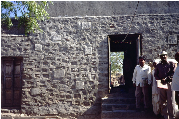
Fig. 41 Engineer, masons and home owners with retrofitted stone masonry home. Through-stones are visible (photo: S. Brzev)
