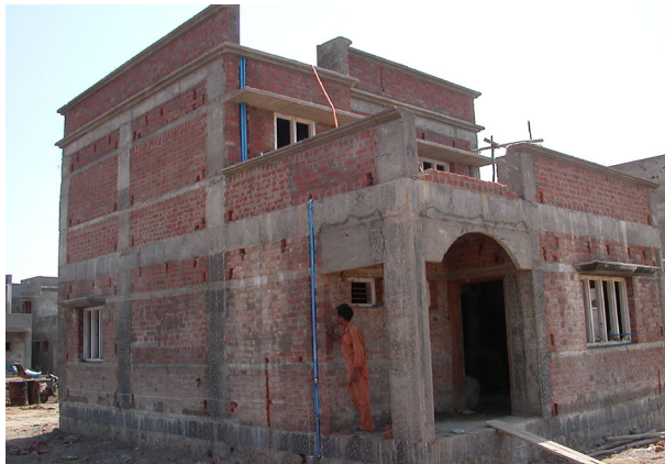
Fig. 53 Two-storey masonry house under construction in Bhuj after the 2001 earthquake with strengthening elements of reinforced concrete that exceed IS 4326 requirements (photo: author)
