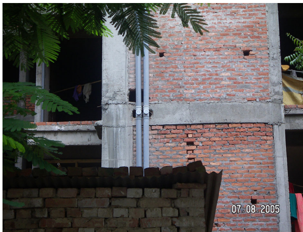
Fig. 64 Pipes perforating the beam of a reinforced concrete frame near the beam column joint in the city of Kanpur in 2005 (photo: C. K. Jain)
