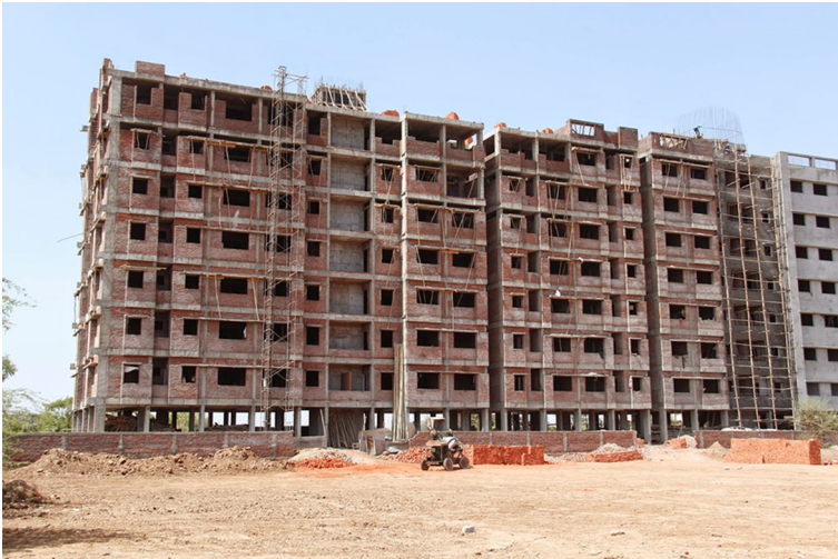
Fig. 65 Multi-storey apartment building under construction in a city in India (photo: author)
