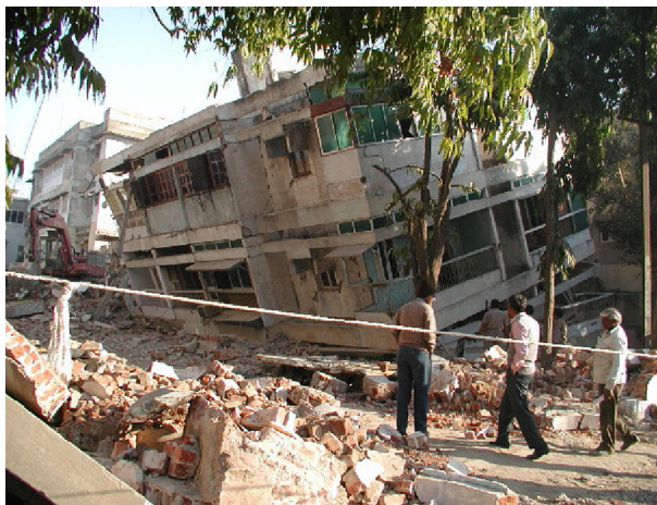
Fig. 43 One of the about 130 multi-storey buildings that collapsed in Ahmedabad, more than 200 km from the epicentre (photo: R. Goel)
