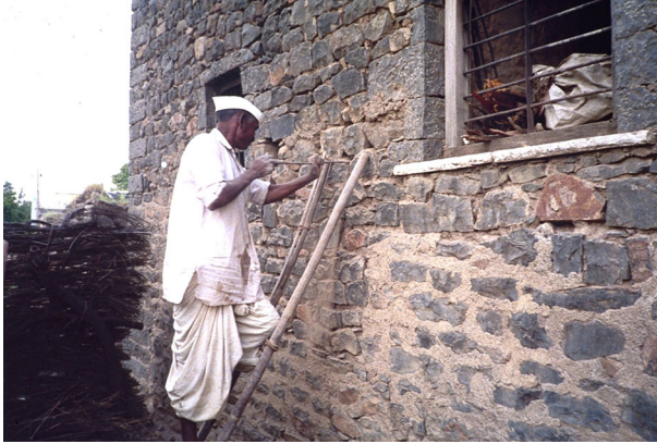
Fig. 40 A mason, in Maharashtra, installing through-stone for retrofitting a masonry house (photo: S. Brzev)
