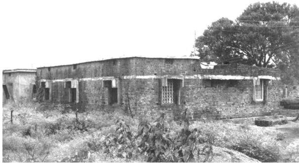
Fig. 52 House with lintel bands in Killari village near the epicentre of Latur earthquake (photo: author)
