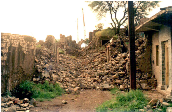
Fig. 5 Collapsed random rubble construction blocks village road in Latur (courtesy: NICEE)
