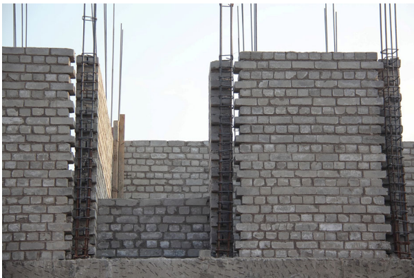
Fig. 55 Confined masonry under construction at IIT Gandhinagar campus, illustrating the masonry walls and tothing (photo: S. Brzev)
