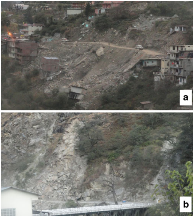
Fig. 6 Landslides occurring along the road corridor: a a large rock-cum-debris slide damaging the houses and the road; b a rock slide blocking the road partially
